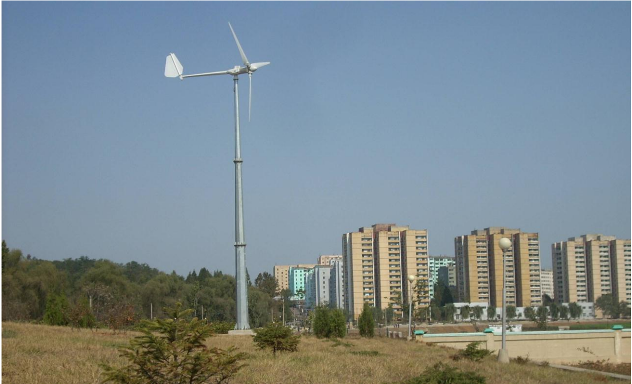
Commercial 5-kW wind turbine as part of a hybrid (wind-PV) electricity backup system for the hospital at Unjong County.
